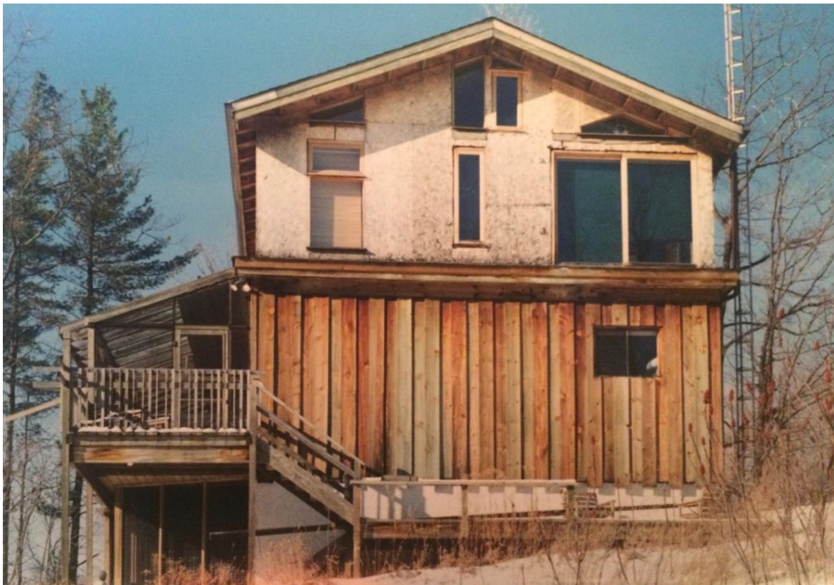
Figure 23 - Side view of the cottage structure c. 1988. The upper floor is incomplete. By permission of the Ferguson family.
