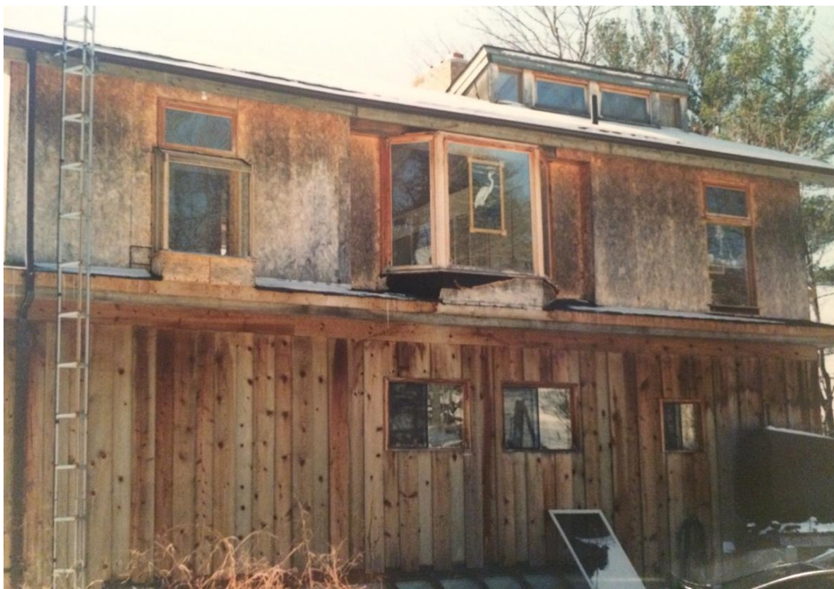
Figure 22 – Rear view of the cottage structure c. 1988. The second floor is incomplete. By permission of the Ferguson family.
