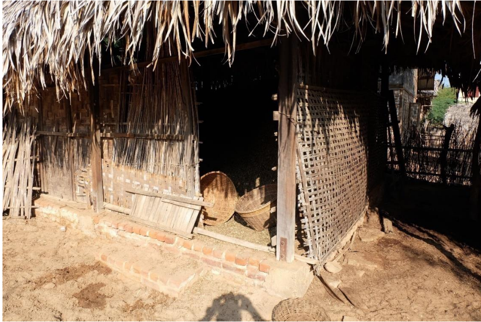
Figure 4.39. Hpauk Sein Pin eastern cow shed fodder storage (Courtesy of Talis Talving-Loza and the IRAW@Bagan Project).
